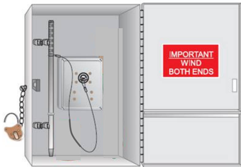
Emergency Operating Lock (EOL) cabinet
