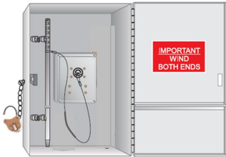
Emergency Operating Lock (EOL) cabinet
