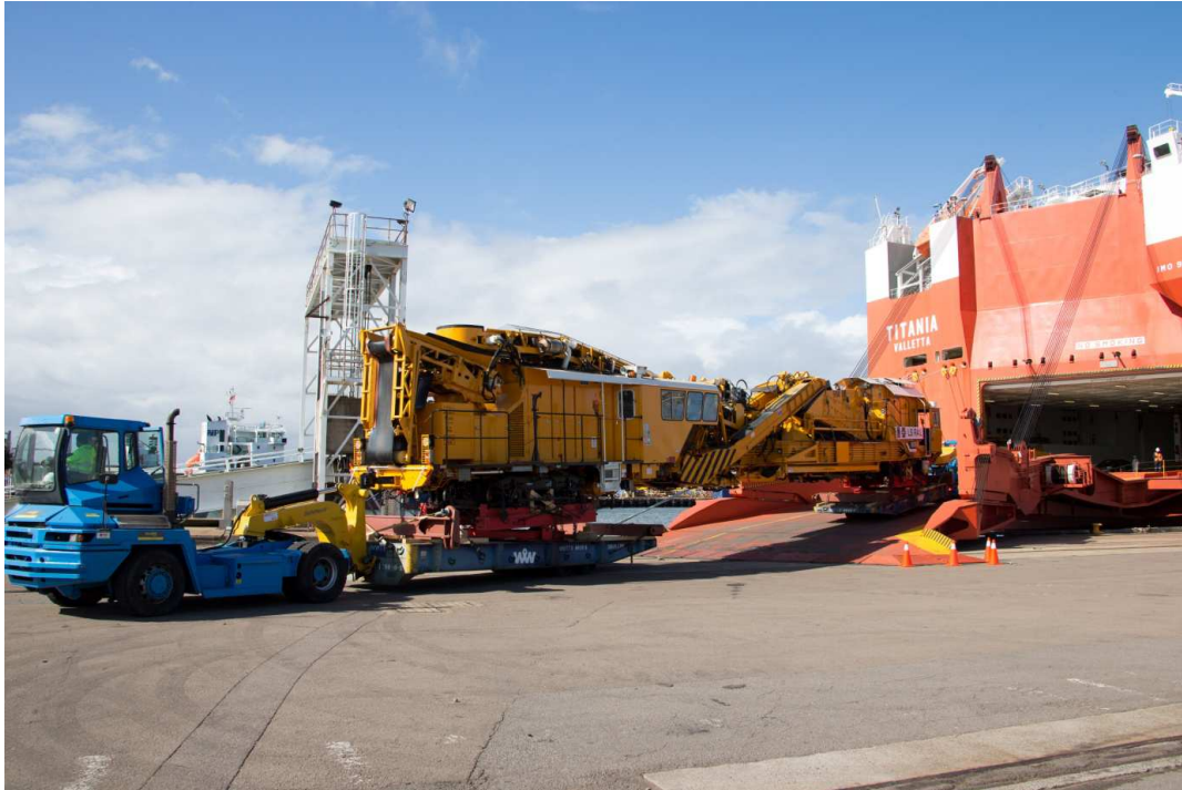
Caption: The LS Rail ballast cleaner arrived at Newcastle Port yesterday and will commence operations in September on the Hunter Valley Coal Network.
