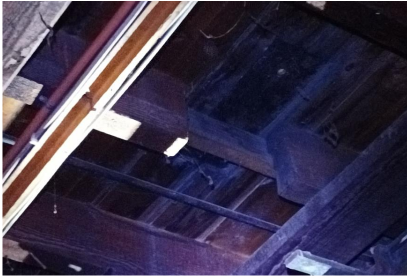
Figure 3-26: Missing middle section of timber beam of first floor
