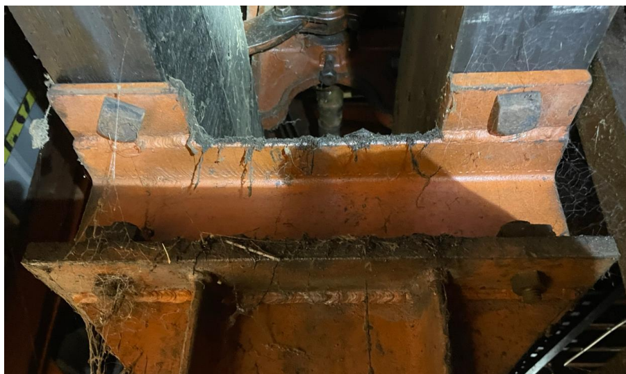
Figure 3-40: Internal steel lever frame supporting first floor elements
