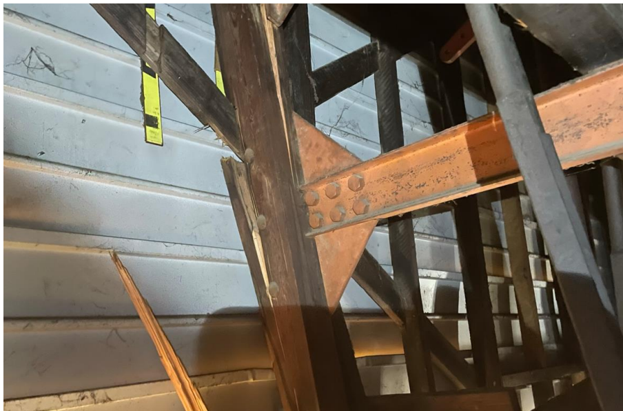
Figure 3-24 Structurally failed members due to impact collision
