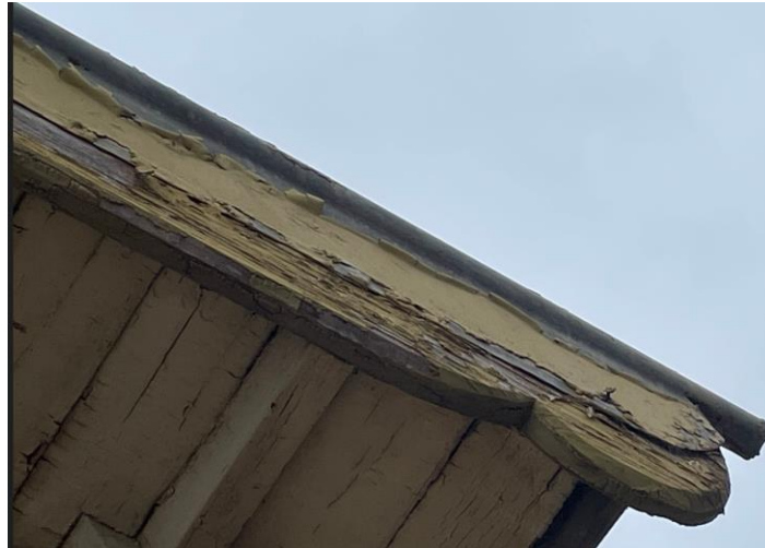
Figure 3-13: Deteriorated fascia member
