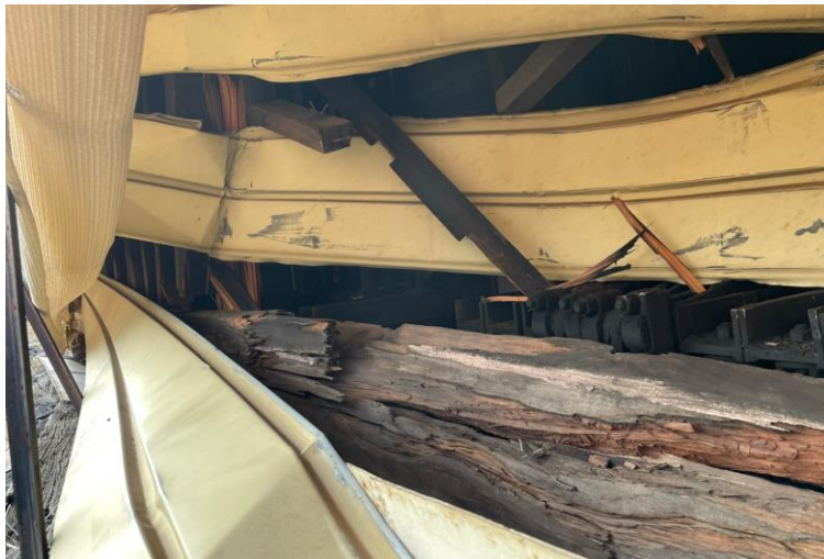
Figure 3-5: Section of external cladding that has been damaged beyond repair.
