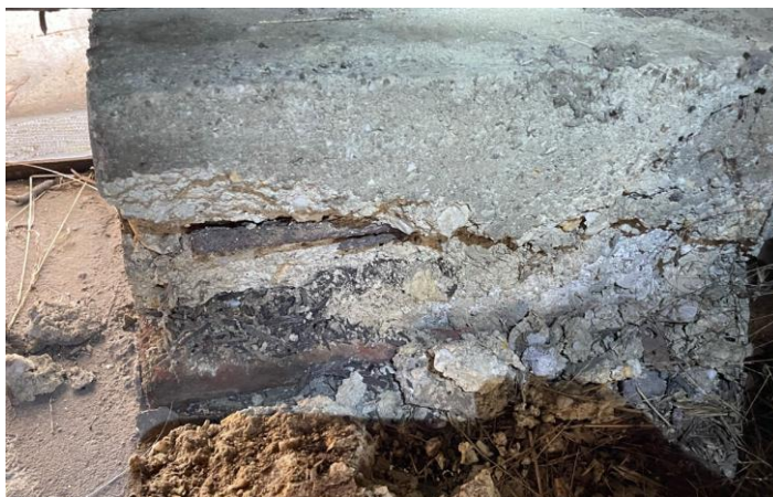
Figure 3-32: Missing piece of the concrete footing
