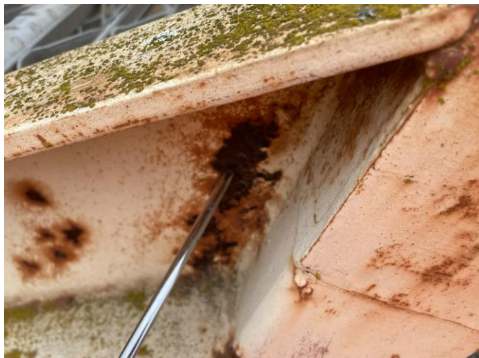
Figure 3-15: Pitting corrosion on one of the PFC members on the external staircase
