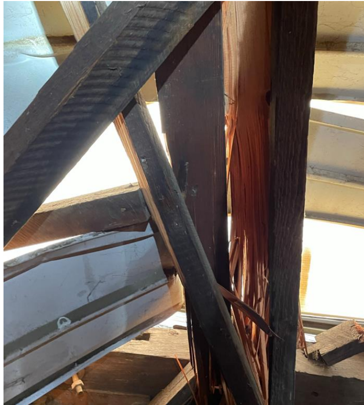
Figure 3-23: Structurally failed column due to impact collision
