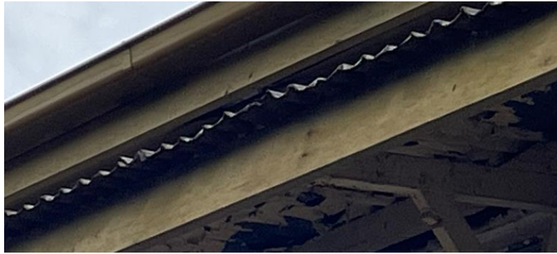
Figure 3-9: Deformed section of the roof sheeting on the lower portion of the roof
