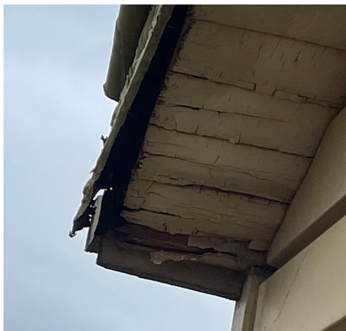
Figure 3-12: Disconnected fascia member and deterioration of the roof lining
