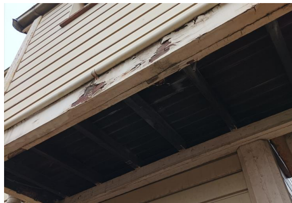
Figure 3-20: Split in external beam supporting first floor toilet
