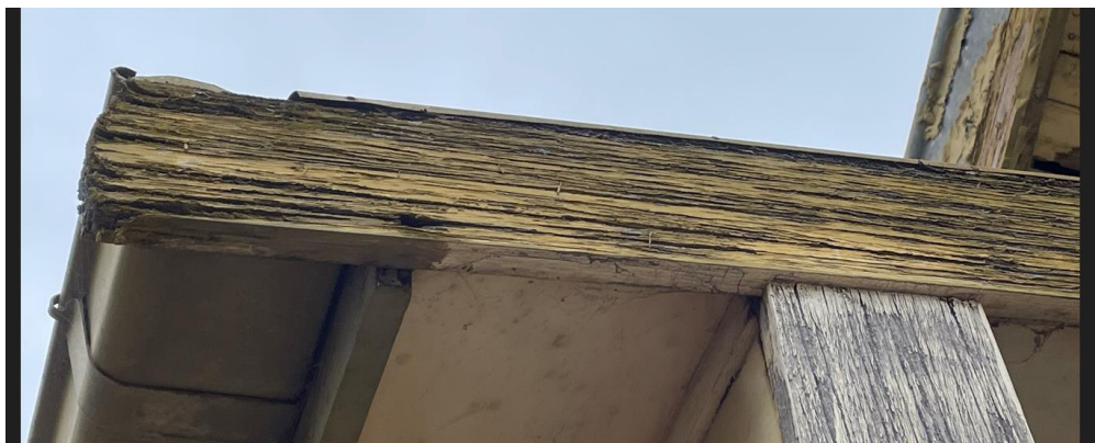
Figure 3-11: Significant splitting and deterioration of the fascia member
