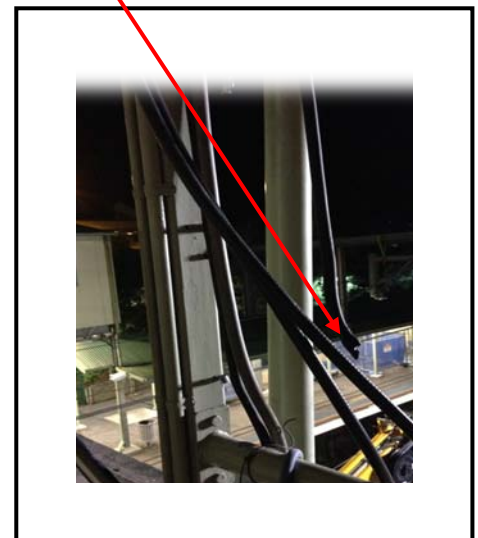
Photograph showing the end of the cut cable
